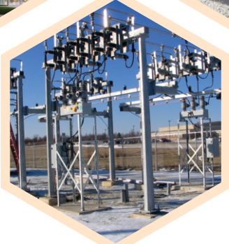
SUB STATION UP TO 132 KV
